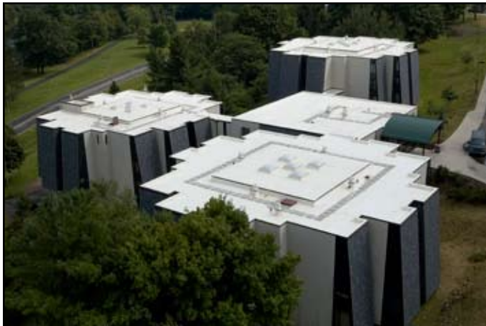
Mid-State Industries, Ltd. removed the existing steep concrete shingle roofs on eight dormitory buildings at the State University of New York (SUNY) and replaced them with 352 squares of DaVinci Slate synthetic roofing tiles.
